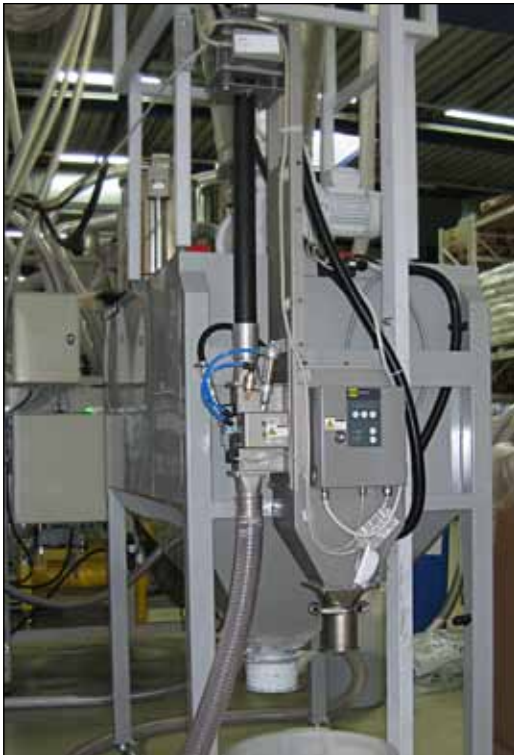
GF metal separator installed in a vertical conveyor pipe
